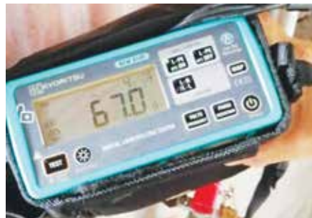
Measuring the earth loop impedance of MSB and transformer star point – reading 67 ohms and fault current 4 amps.
