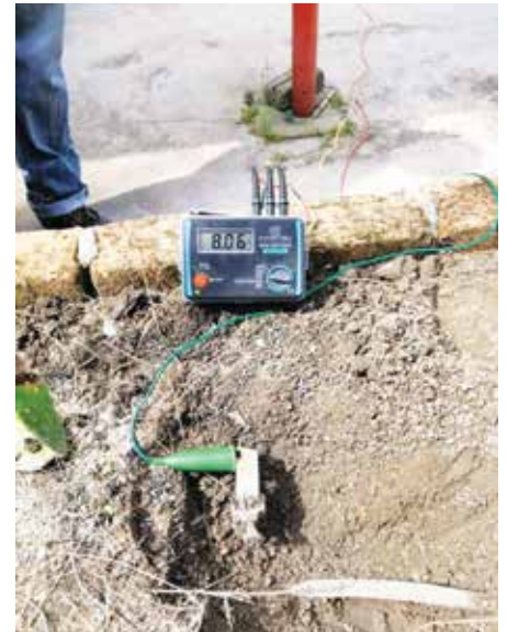
Measuring Re at Consumer's MSB earth electrode – by Fall Potential Method using earth resistance tester.
